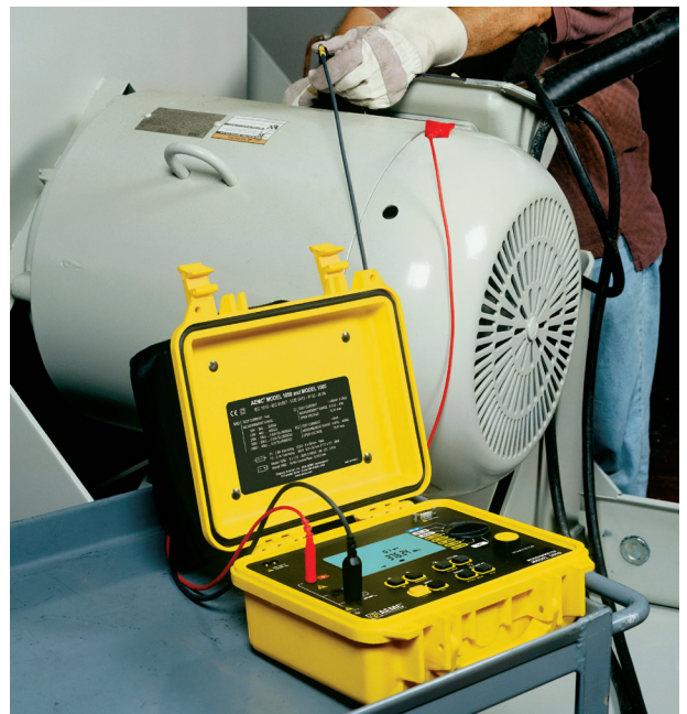
Photo 1. A worker performs an insulation resistance test on a 50-hp 480V motor.
